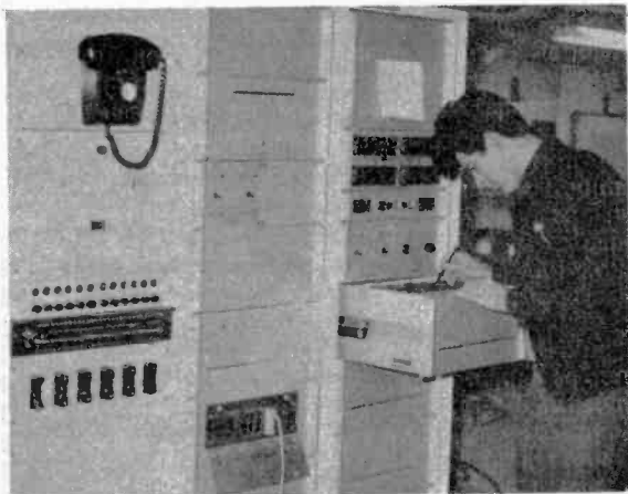
This is the logic equipment for the steering of Aerial No. 2. Technician John Austin is seen here inspecting one of the logic board modules.
